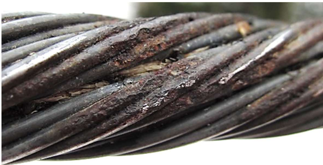
Wire breaks due to corrosion
