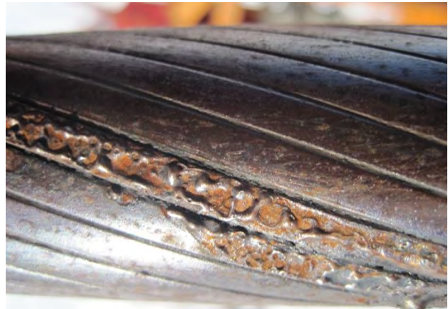
Figure 2-11: Lightning strike at locked coil rope
