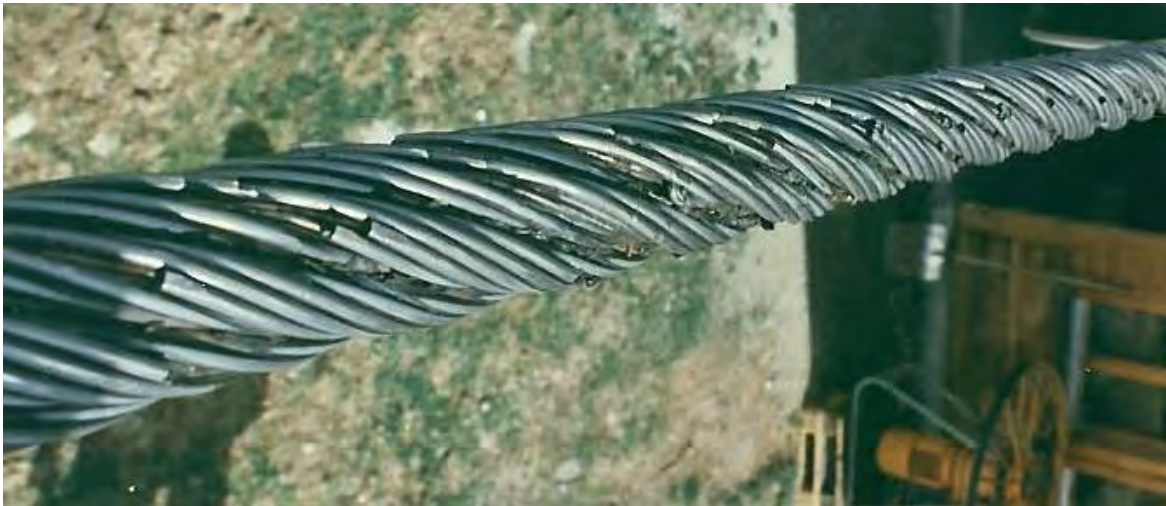
Figure 2-2: Damages of slipped mounting clamp
