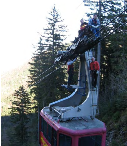
Figure 3-8: Visual inspection of track ropes on a ladder, a platform, a chair and the carrier truck
