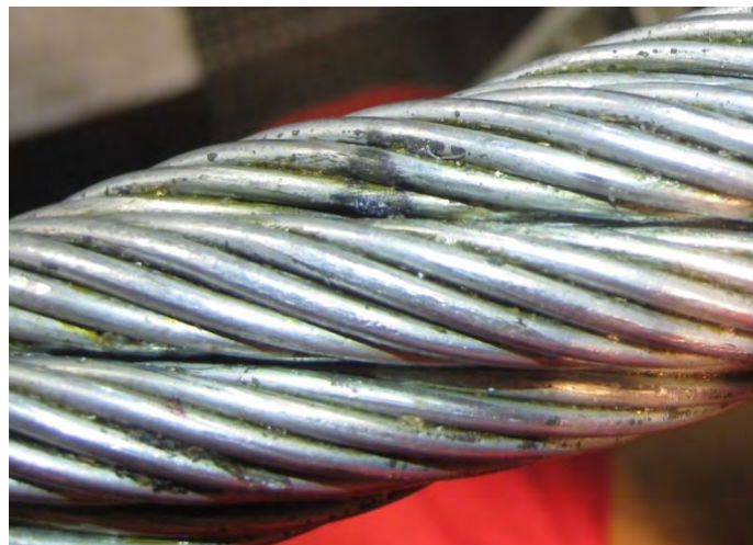
Figure 4-1: Lightning strike bluish discoloration
