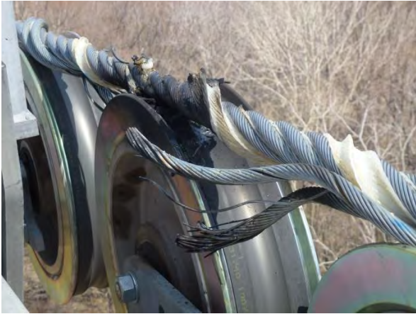
Figure 2-6: Damage by current flow
