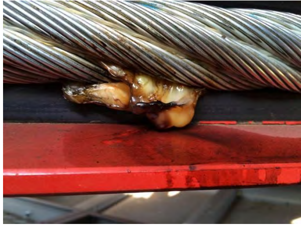
Figure 2-7: Damage by current flow
