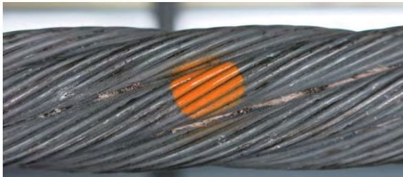
Figure 4-23: Corrosion 1.0 x strand diameter
