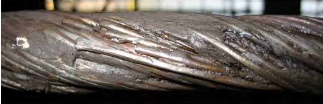
Picture 13: Very dirty rope – inspection not possible!
