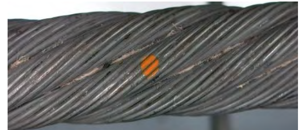
Figure 4-24: Corrosion 0.5 x strand diameter
