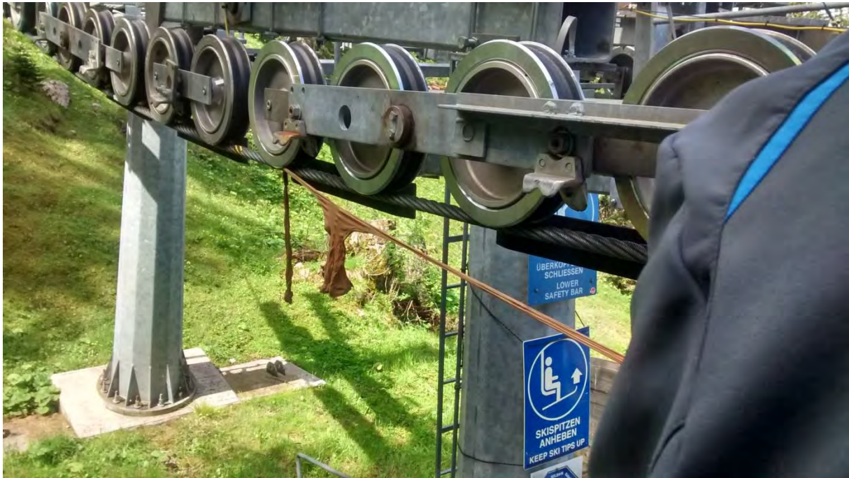
Figure 5-19: Nylon stocking gets stuck on the rope and is dragged into the roller battery
