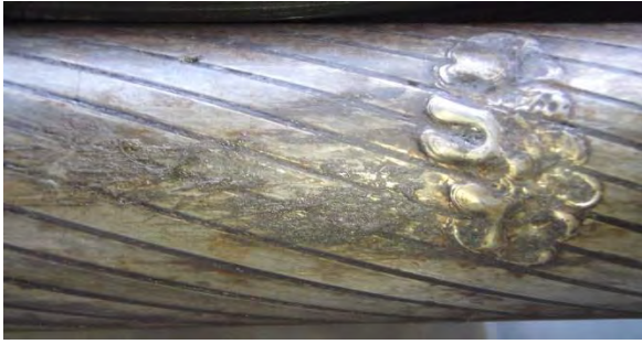
Figure 2-14: Point of impact at the underside of the rope
