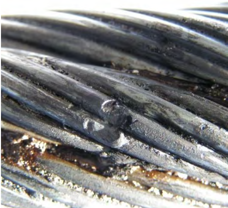
Figure 2-4: Damage by current flow
