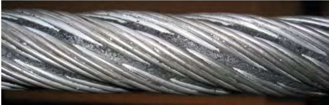
Picture 14: Dirt in strand touching zones – hard to inspect
