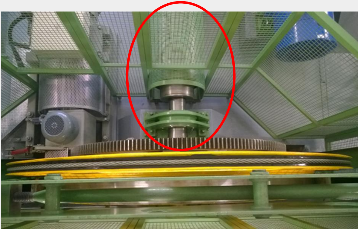
Electric Main Drive
