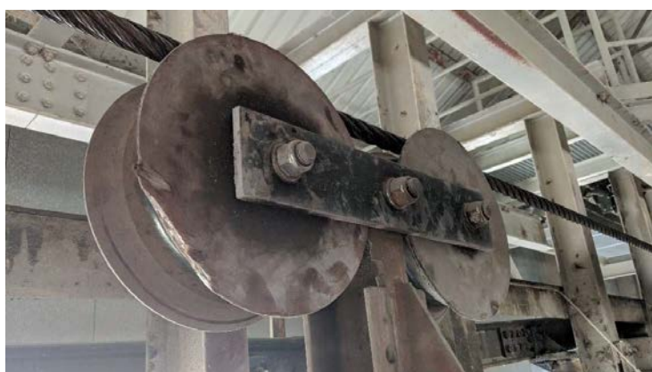
Roller Damages seriously damage the rope
