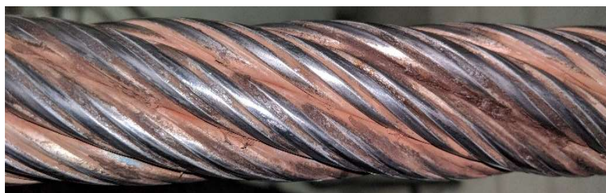
Corrosion induced by friction between touching strands
