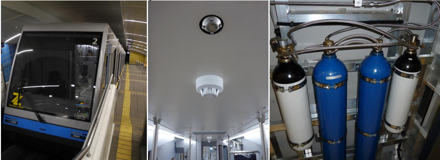
Automatic fire detection and extinguishing systems
