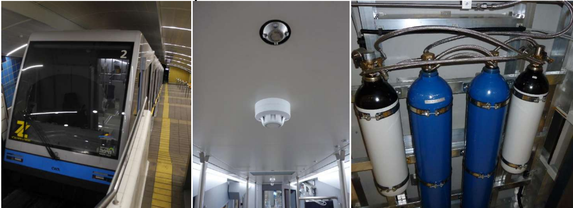
Automatic fire detection and extinguishing systems
