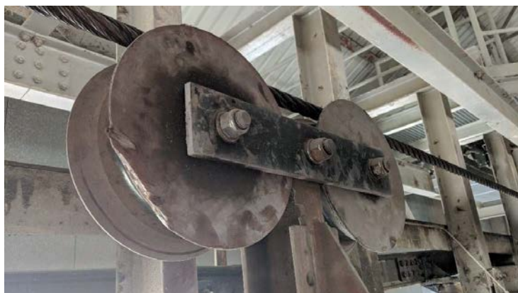
Roller Damages seriously damage the rope
