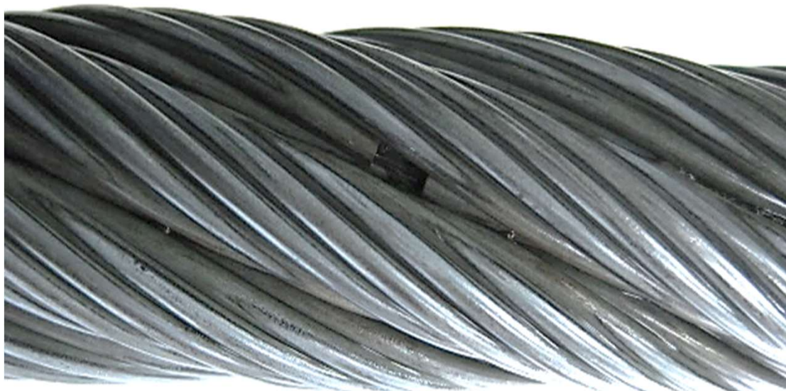
Common wire break due to bending cycles
